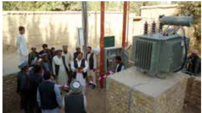
Power line supply, Khuja Sabz Posh, district Faryab
